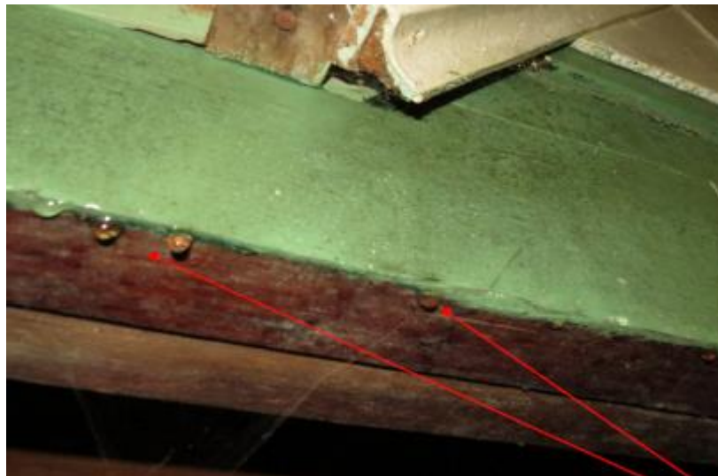
Condensation importante Significant condensation
