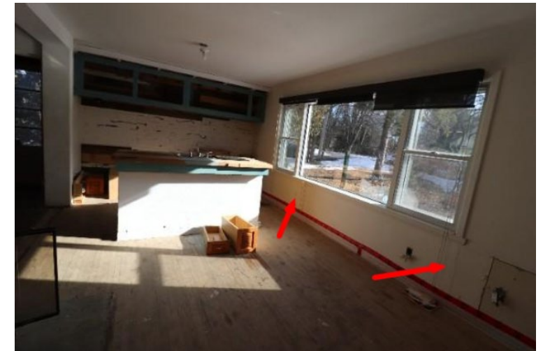
signe de cisaillement de la structure signs of cracks in the structure
